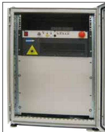
Integration in an electrical cabinet
